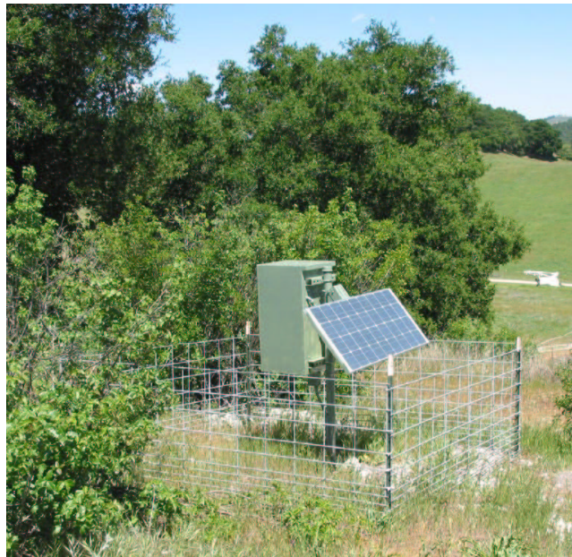
Figure R3. Solar panel, power supply and telemetry system for the PBO site P526, located on the Ramage Ranch.
