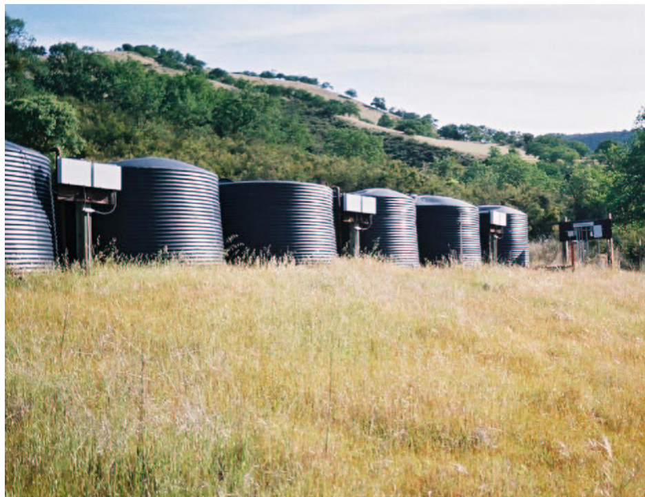
Figure H6. View from the side of the ridge looking NE towards the water tanks. The power panel is visible on the far right and Red Rock hill is in the background.
