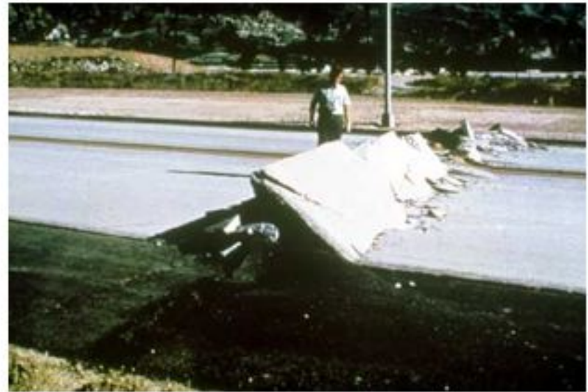
Roadway compression 23", most damage within 6 miles of epicenter
